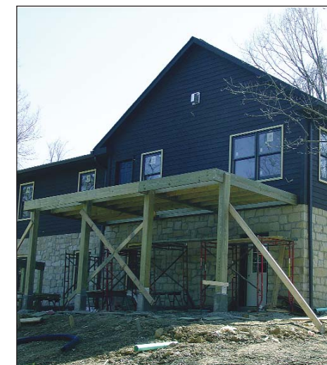
Construction continues on the three new 8-bedroom cottages. The cottages are expected to be completed by July 2008.
